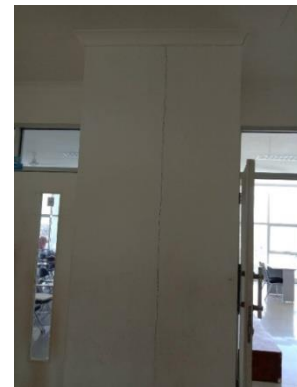
Figure 3. Cracks in Building E
