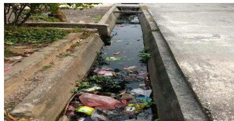
Figure 4. Drainage incapable of draining water runoff
