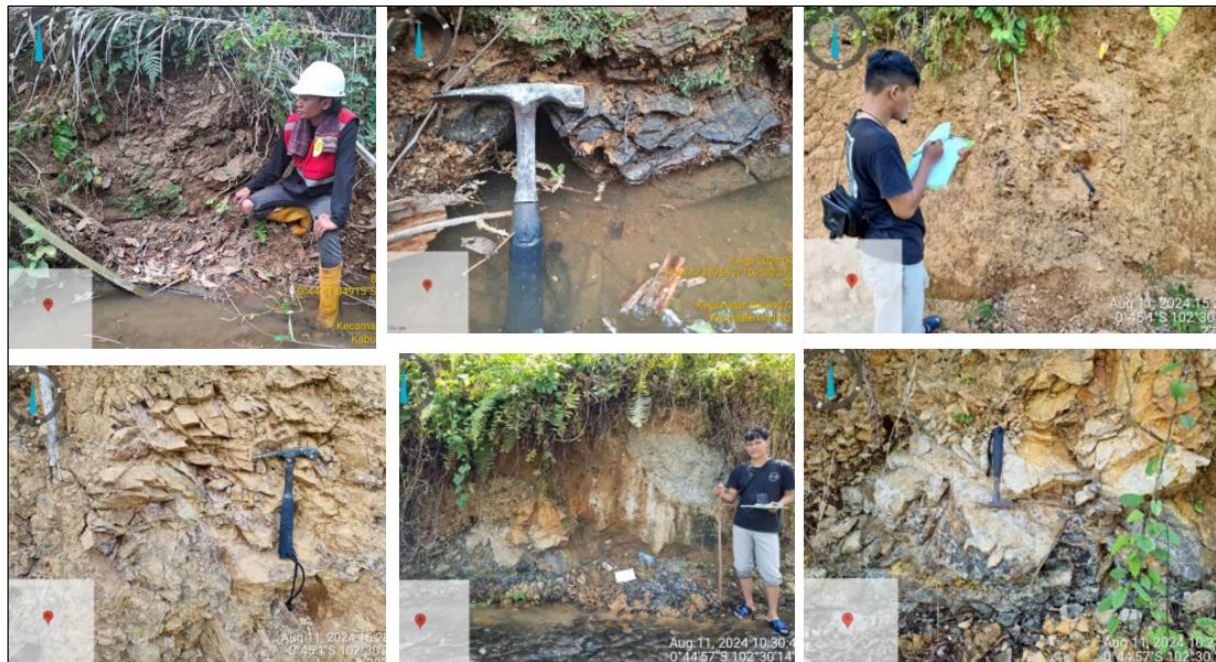
Fig 4. Location and Condition of Slopes in the Andesite Quarry Area
