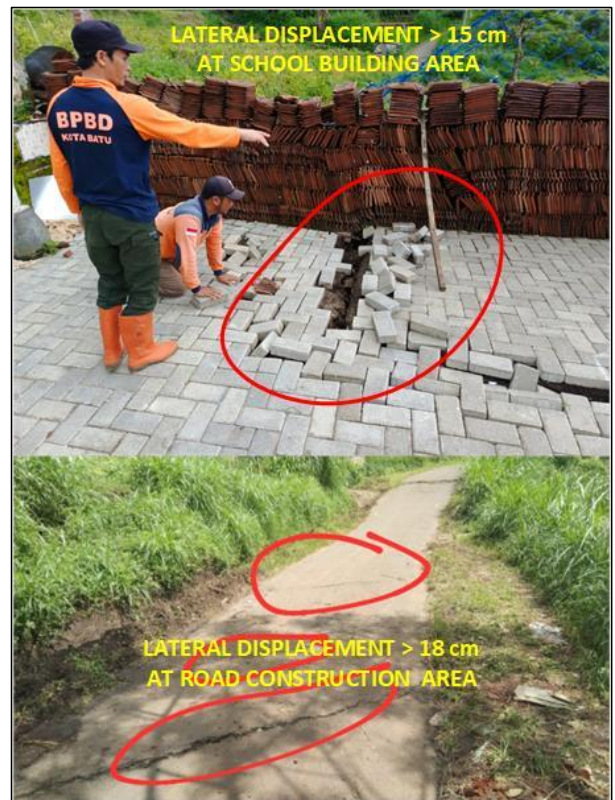
Fig. 5. Existing width of the cracks or fracture occurred
