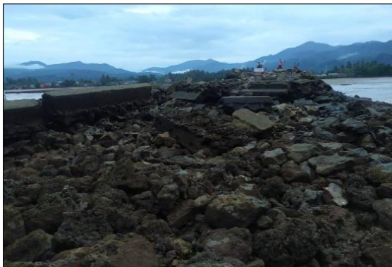
Fig 3. The Outer End Condition of Tinobu Port's Causeway Has Collapsed
