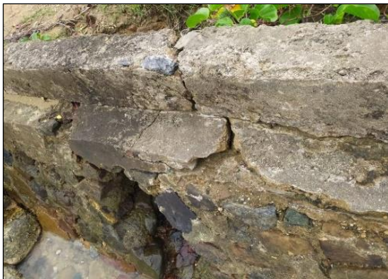
Fig 2. The Damage Condition Occurring on Almost the Entire Body of Tinobu Port's Causeway
