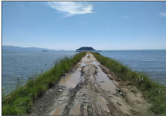
Fig 1. Condition of the Surface of Tinobu Port's Causeway
