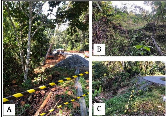
Fig 1. Several landslide alongside the cross-province road of BBSNP
