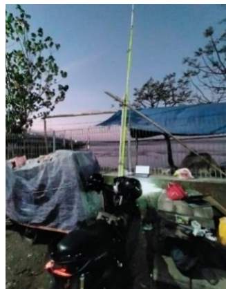
Figure 6. LoRa Gateway installation site on Suramadu bridge
